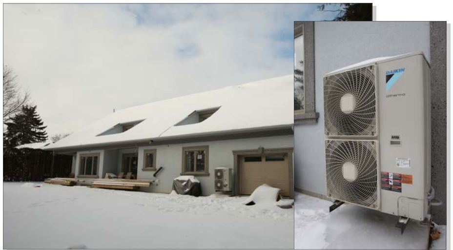
The 4,350-square-foot (plus 2,000 square feet in the basement) home, which also includes a four-car garage and a 12x26 foot storage area above the garage, was situated for maximum solar gain and incorporates south facing windows.
